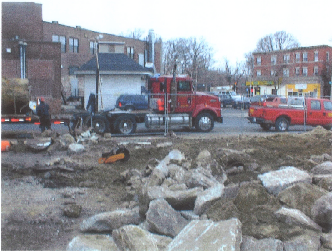
Photo 5: Last UST is prepared for transport to disposal facility: photo taken on 3/9/06 while facing west.
