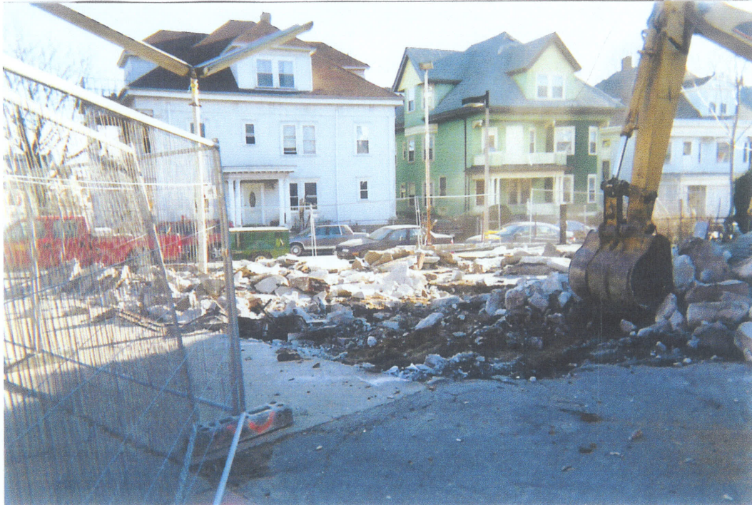
Photo 1: Excavator removes the concrete broken up earlier with a hoe-ram: photo taken facing east on 3/7/06.
