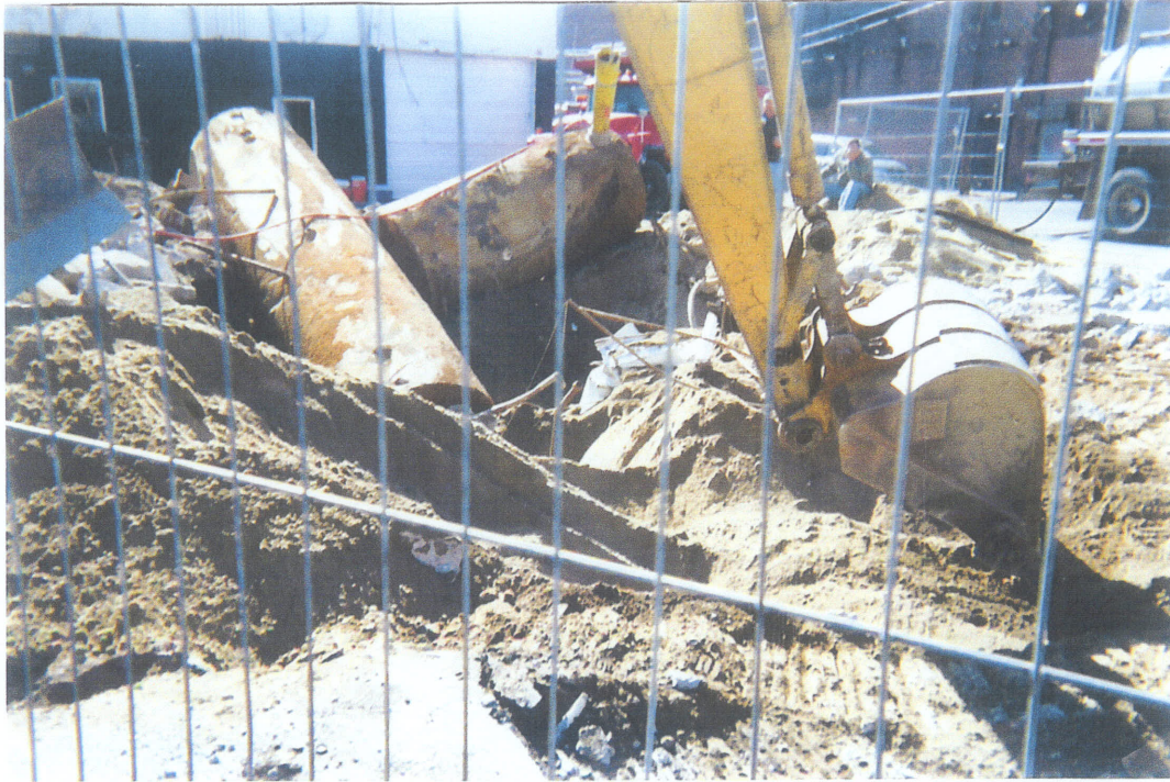
Photo 3: USTs are unearthed, vented, and dry ice is added to inert: photo taken facing north on 3/8/06.
