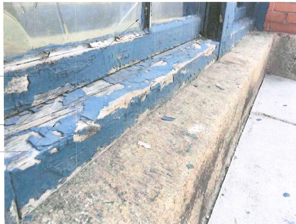
DAMAGED + ROTTING WOOD SILL
