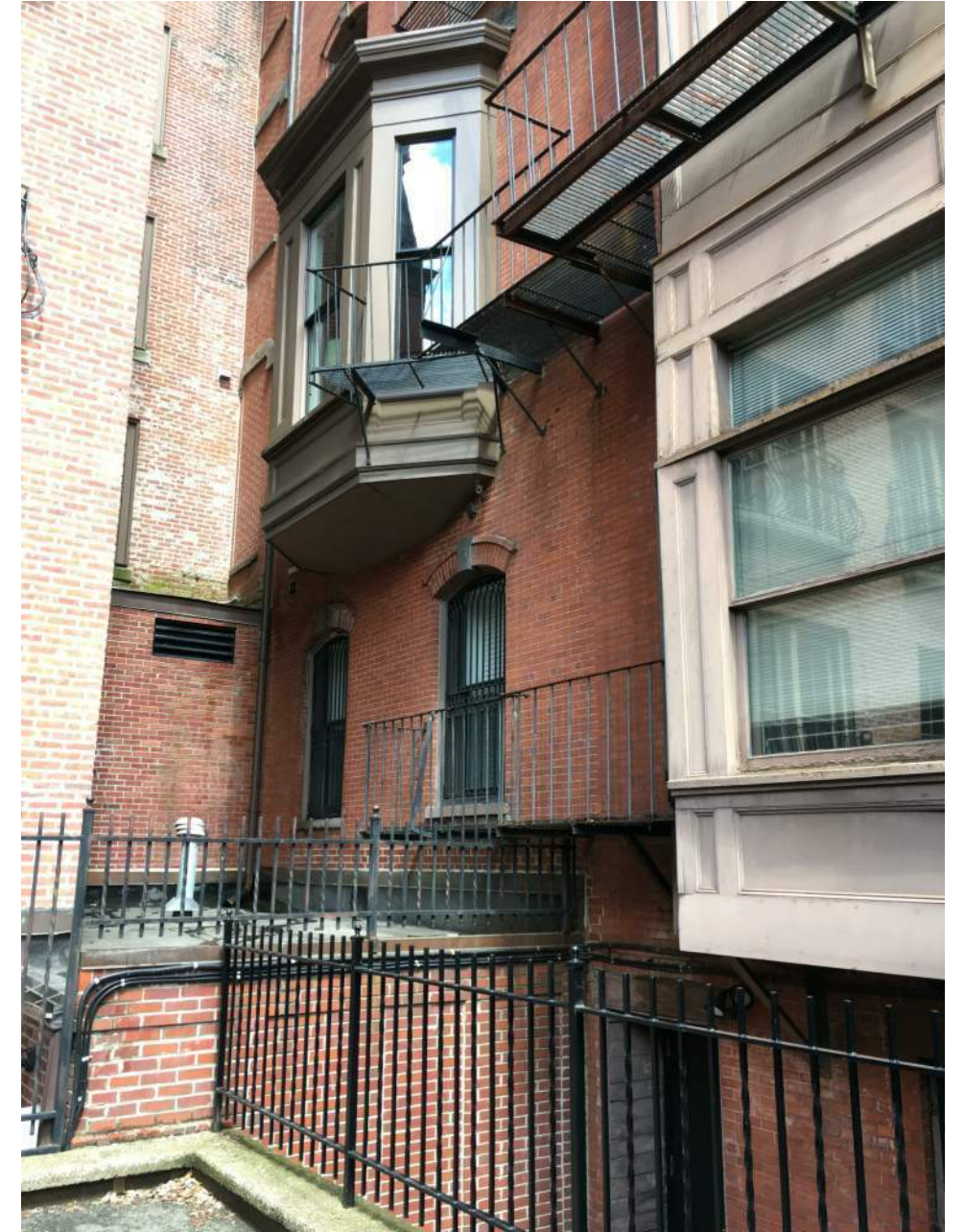
MATCHING SINGLE STORY ORIEL AT NEIGHBORING PROPERTY
