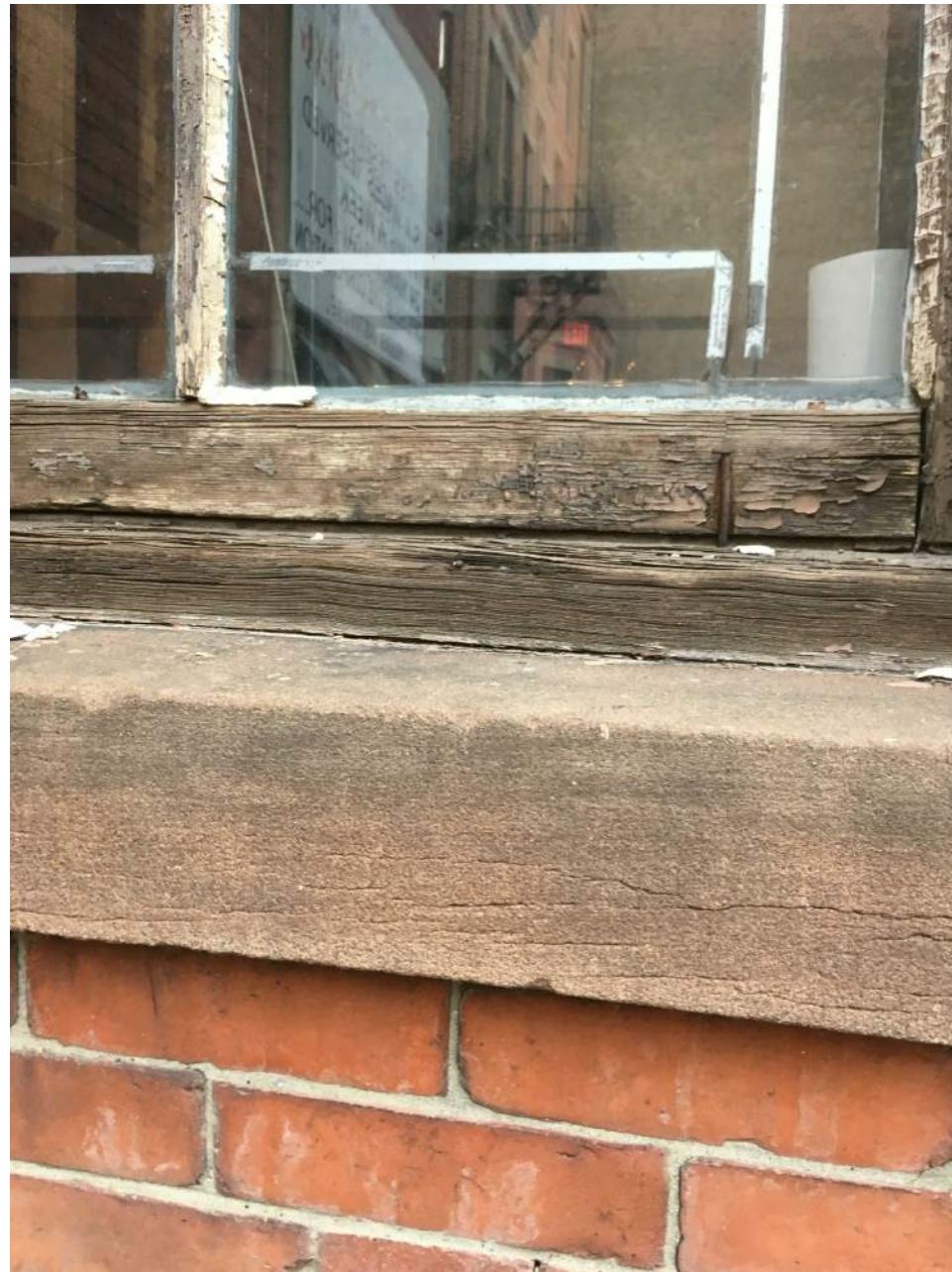
EXISTING WOOD WINDOWS TO BE REPLACED. STONE SILLS TO BE REPAIRED AND RESTORED, AS REQUIRED.
