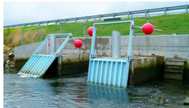
Example: Self Regulating Tide Control Gates
