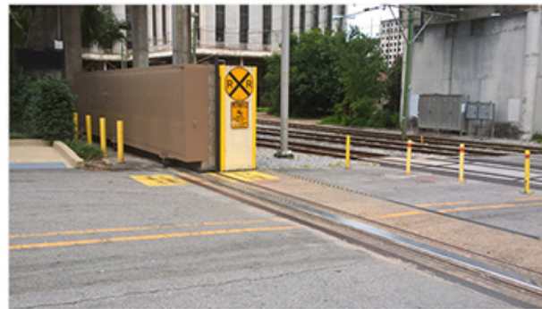
Example: Deployable Barrier, New Orleans, Louisiana. Designed by U.S. Army Corps of Engineers.
