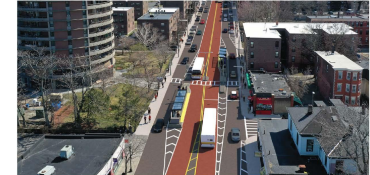
Columbus Avenue dedicated bus lanes, under construction in early 2021. Source: Massachusetts Department of Transportation (MassDOT)
