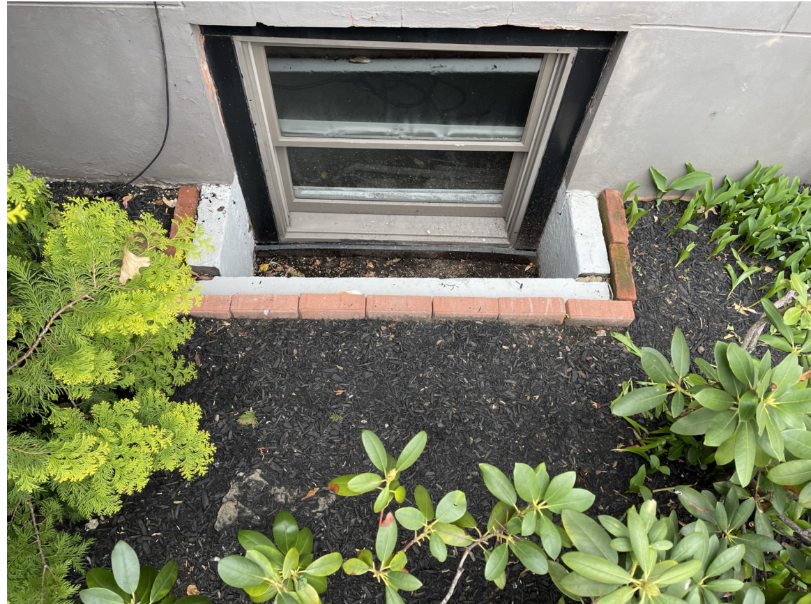
RIGHT BASEMENT WINDOW
