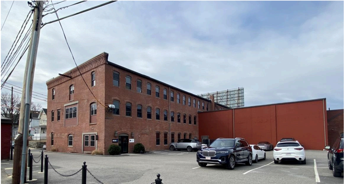
Figure 5. 12 Ericsson St. showing blocked-in window and door openings on the east- and north-facing rear elevations and the concrete-block structure connecting to 12R Ericsson St. Photo by John D. Clemson, March 17, 2023.
