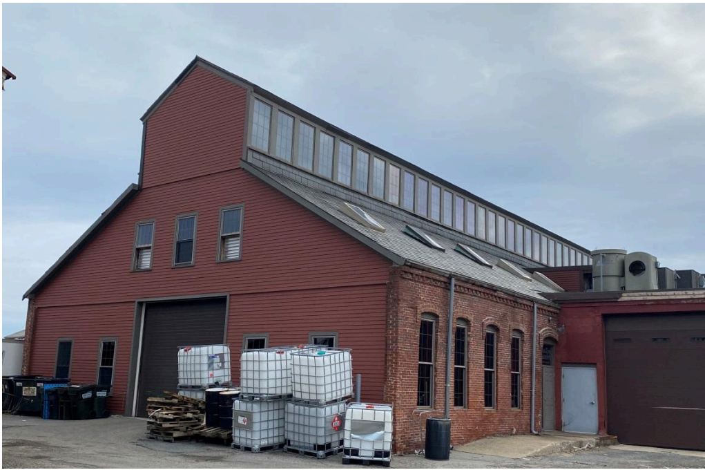
Figure 9. West-facing elevation of 12R Ericsson St. Photo by John D. Clemson, March 17, 2023.
