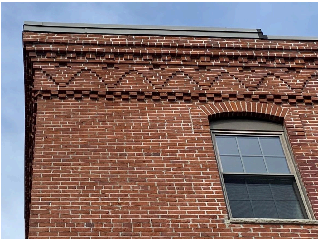
Figure 6. 12 Ericsson St. viewed from the east showing window label and cornice and parapet detail. Photo by John D. Clemson, March 17, 2023.
